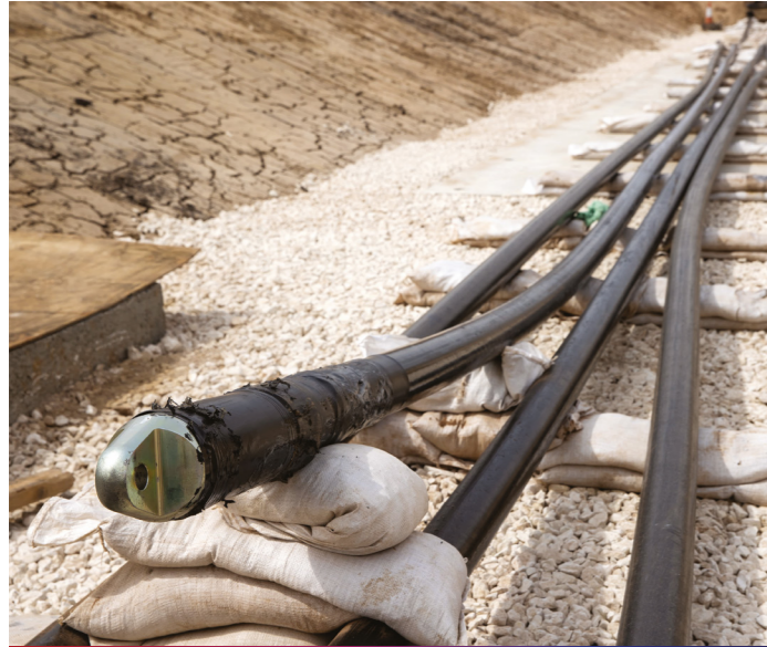
Onshore cable testing success
