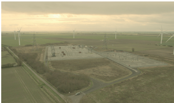
Bicker Fen substation
