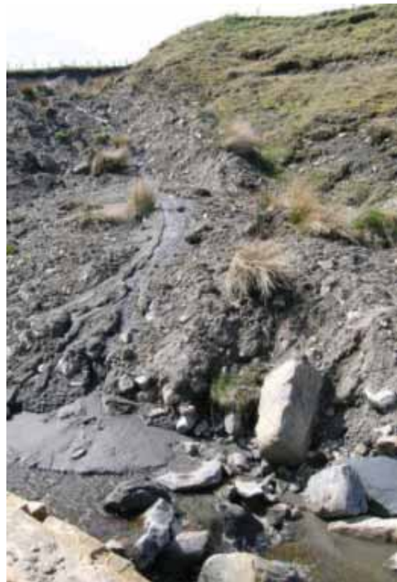
Soil erosion caused by runoff
